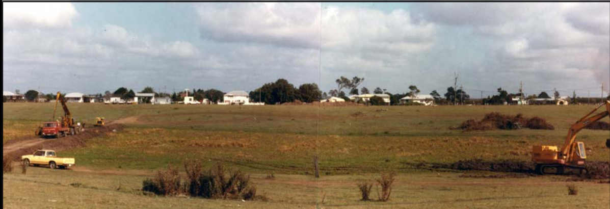
bun02807 Beginning the excavation of Lake 1 at the Botanical Gardens area, Nov 1983
