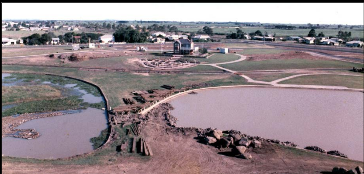
bun02815 Start of the boardwalk construction around the lakes March 1986. Hinkler House and Rose Garden in background.
